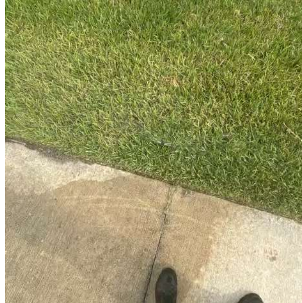
Zone #19 (Clogged Nozzle) - 05-11-26 9:12 am CDT
